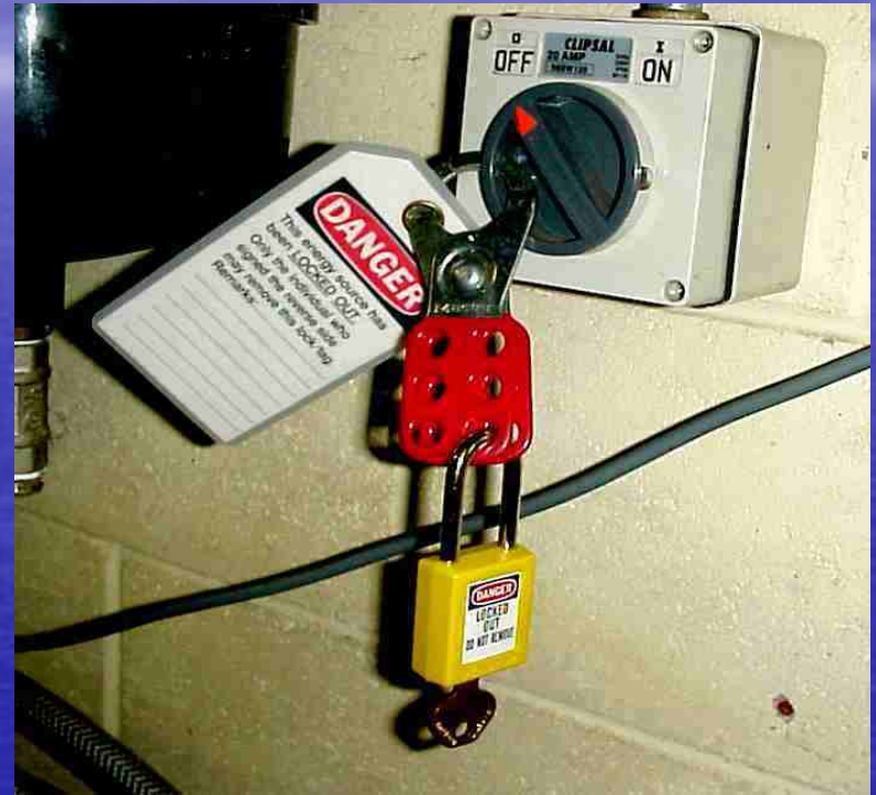
Lock Out / Tag Out Isolation System
