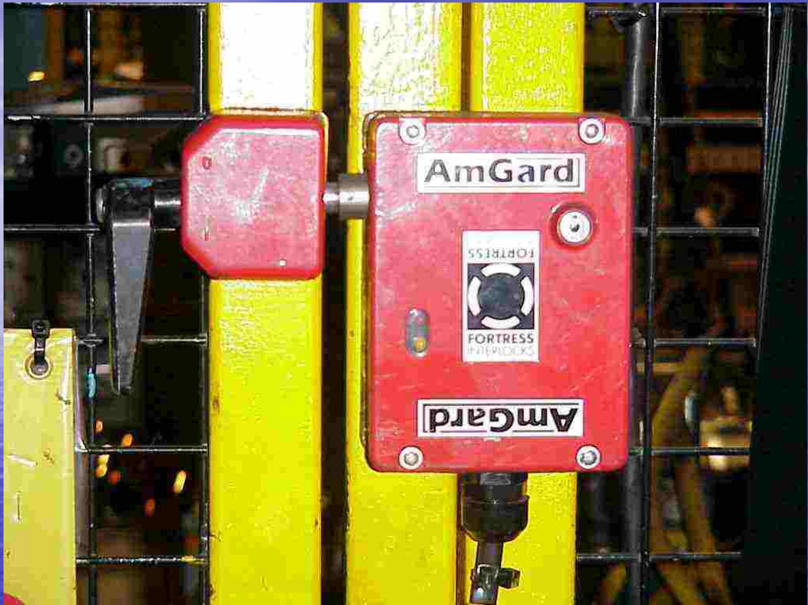
Fixed and Interlocked Barrier Fence Guard
