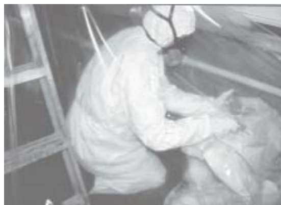
Protection of the worker and the surrounding area is regulated by legislation.
